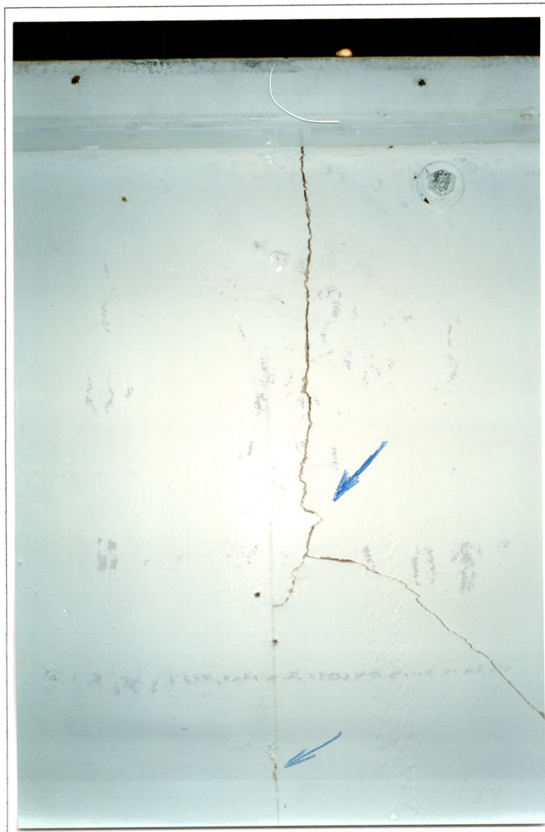
Compartimento da fossa, antepara de vante - Rachaduras horizontais e verticais na antepara. Holding Tank compartment forward bulkhead- Verticals and horizontal cracks in the bulkhead.
