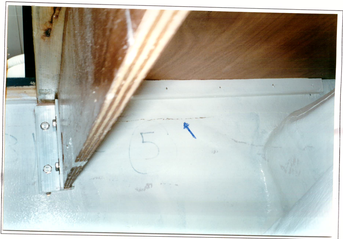
Antepara entre cabines - Rachaduras horizontais. Bulkhead between cabins - Horizontal crack.
