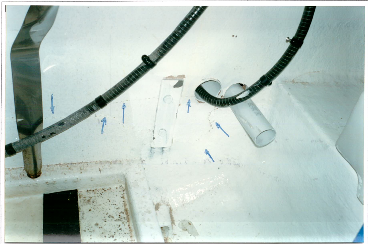
Compartimento da fossa, antepara de ré - Rachaduras horizontais e verticais na antepara. Holding Tank compartment back bulkhead - Verticals and horizontal cracks in the bulkhead.
